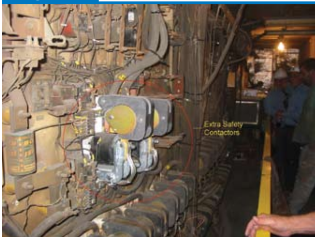
EB contactors installed.
